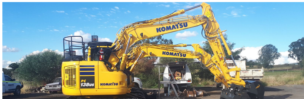
Pictured above: On site, part of the Mulgoa Komatsu PC138US excavators range.
