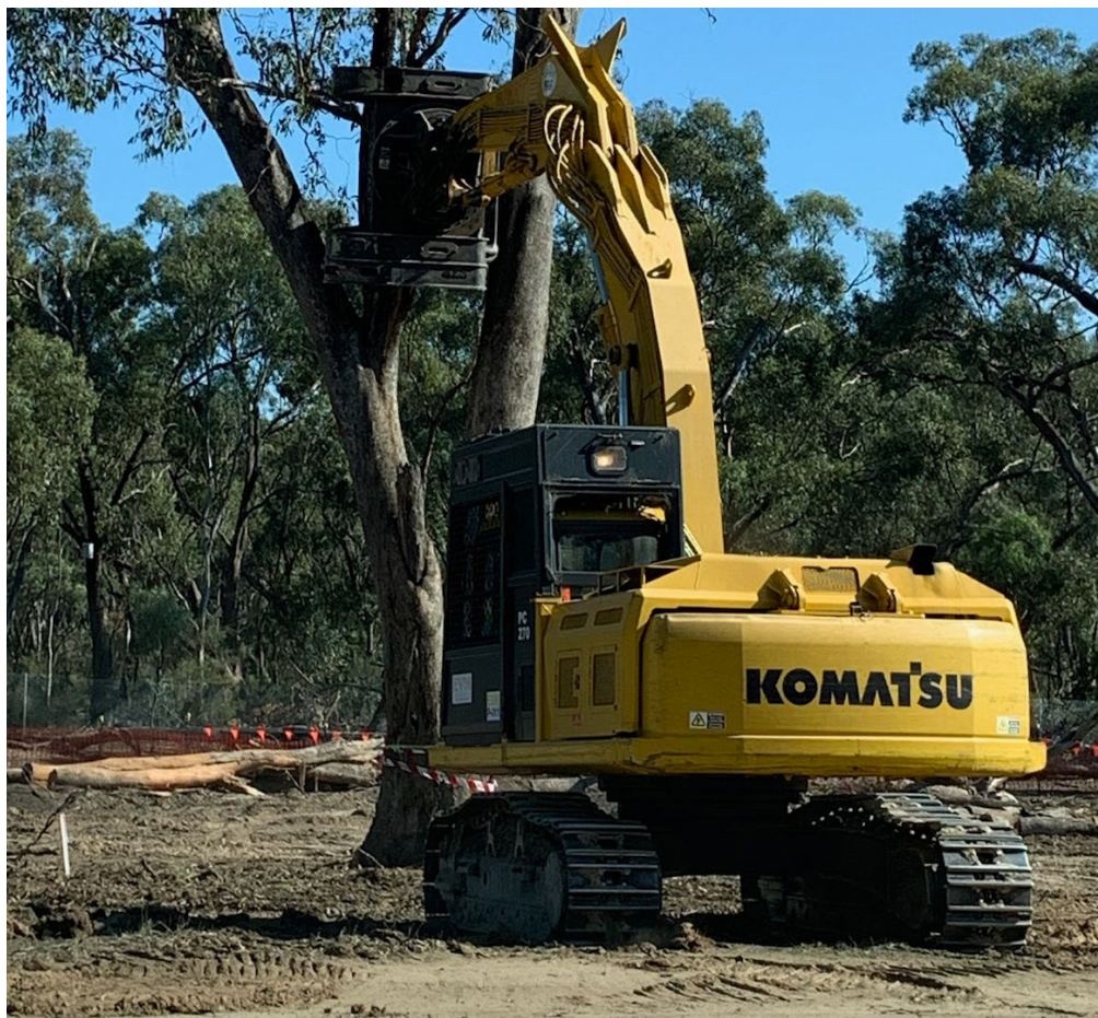
Pictured below: Komatsu PC 270-8 excavator, out in the field with fine touch hydraulic controls, gives its skilled operators the best opportunity to work in highly sensitive areas.
