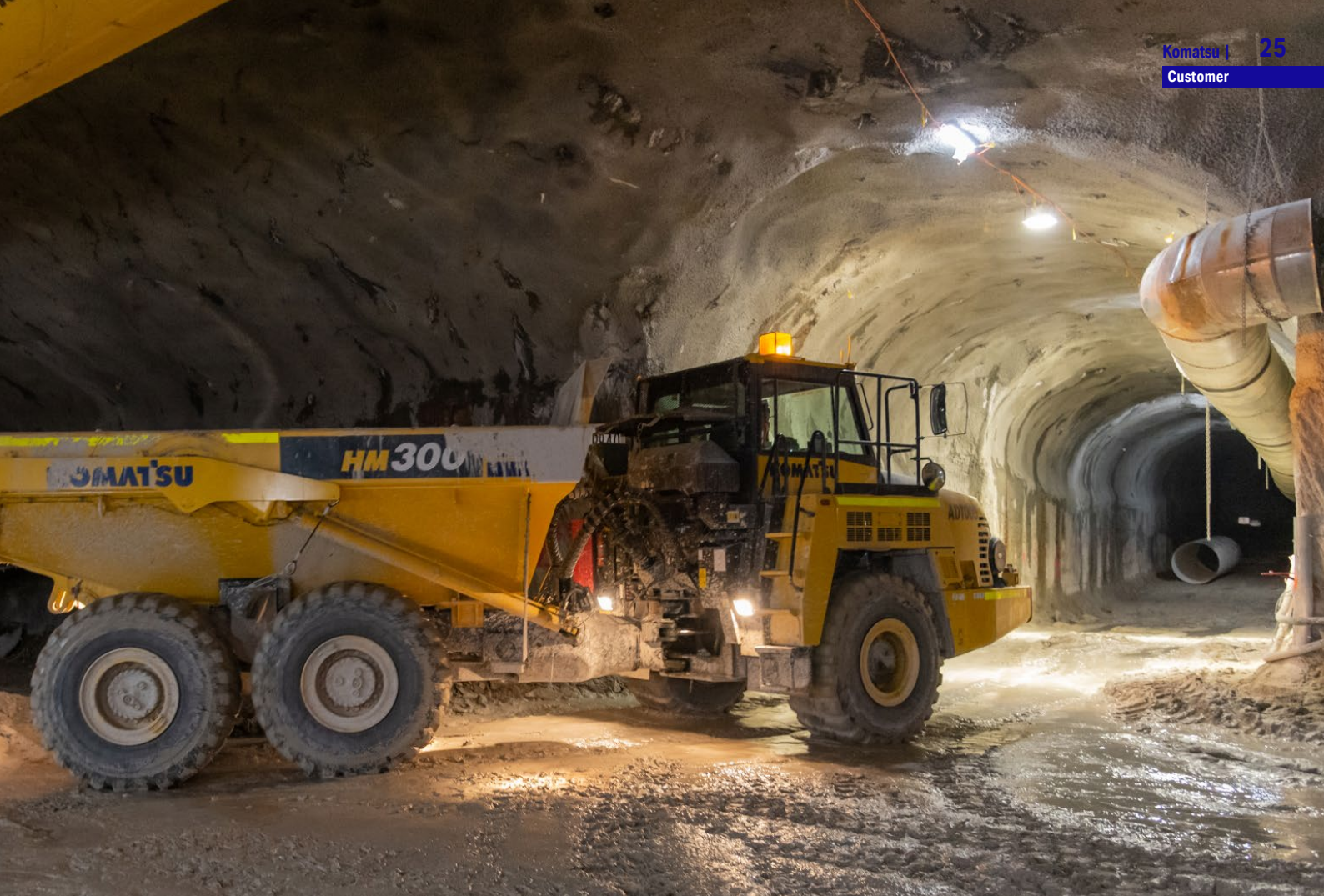
Pictured above: The project is taking advantage of Komatsu's low emissions engines and Komtrax monitoring technology.
