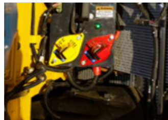
Battery Isolation Single pole, lockable Boschtype battery isolation.
