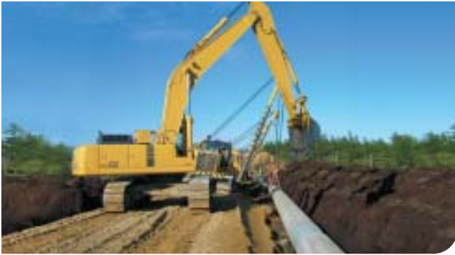
▲ D355C large pipelayer (background) and PC400 medium-sized hydraulic excavator (foreground) deployed for pipelaying in Yamal Peninsula
