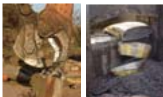
Demonstration test of counterweight dismantling Left: Dismantling using a LaBounty shear; right: dismantling using a guillotine shear
