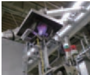
Verification test of the heat-treating furnace at the Awazu Plant
