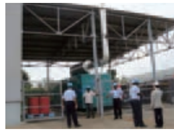
Measurement for exhaust gas emissions from the electrical generator (in Komatsu India Pvt. Ltd.)
