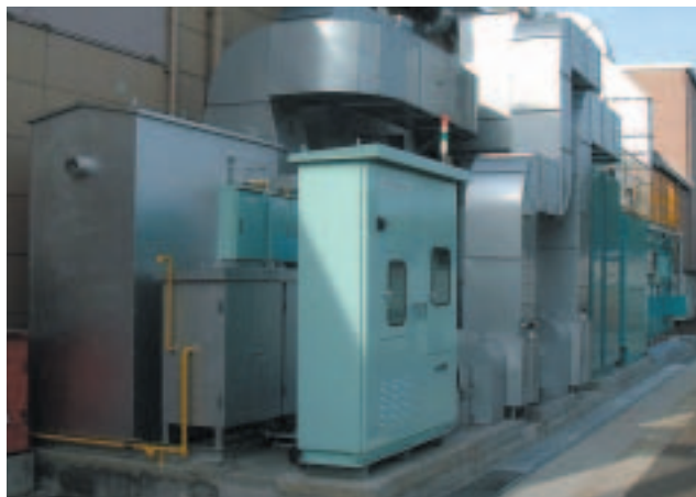
Equipment at Awazu Plant to process VOCs in emitted gases
