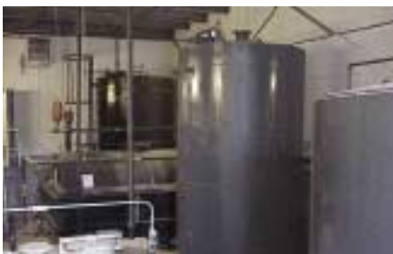
Replacing underground water tanks with above ground ones (indoor installation to protect against snow)
